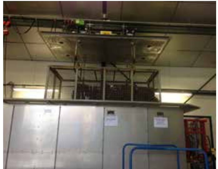
Picture 8: Hot Water Treatment installation (IFV South-West)
